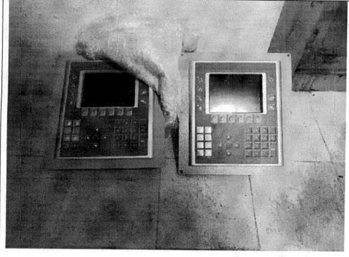
Painel eletronico RIETER – Robos
